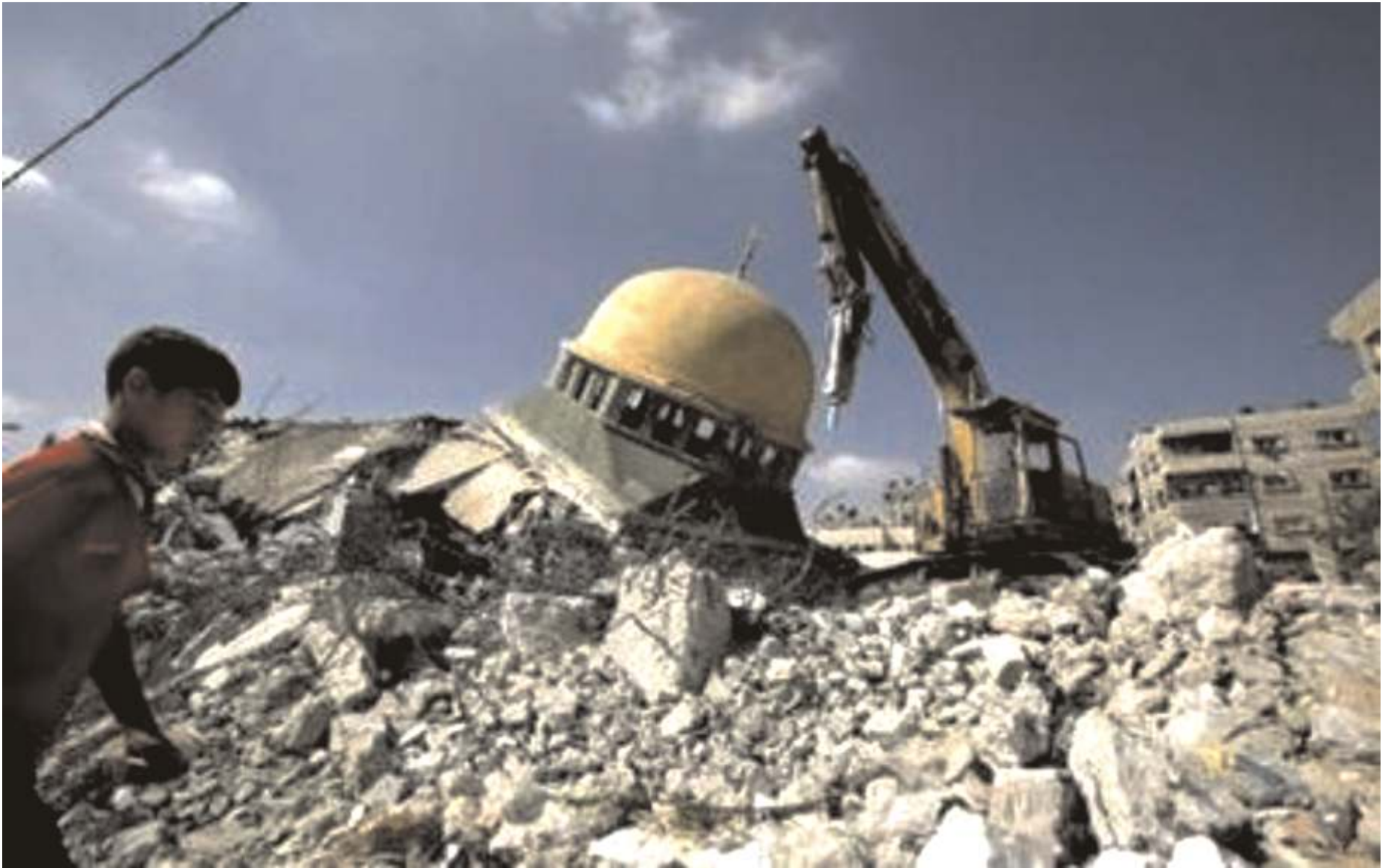
A Palestinian boy walks past the rubble of al-Taqwa mosque that was destroyed by Israel's three-week aggression on Gaza early this year. Gaza remains under total blockade by Israel where people are subjecting of a genocide and are unable to rebuild thousands of destroyed homes and hospitals as a result of the Israeli attacks, July 26, 2009.
